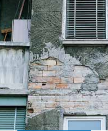
Degraded building façade in need of repair
