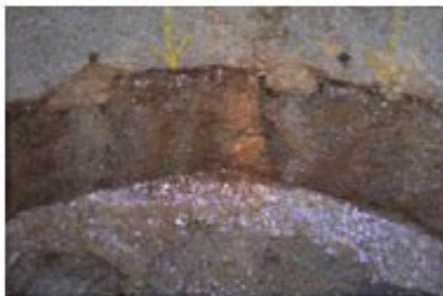
Deteriorating barrel joint with infiltration
